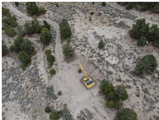
Figure 1 – Aerial footage of a drill pad that will be utilized in the upcoming drill program at Limousine Butte, Nevada To view image please click here
